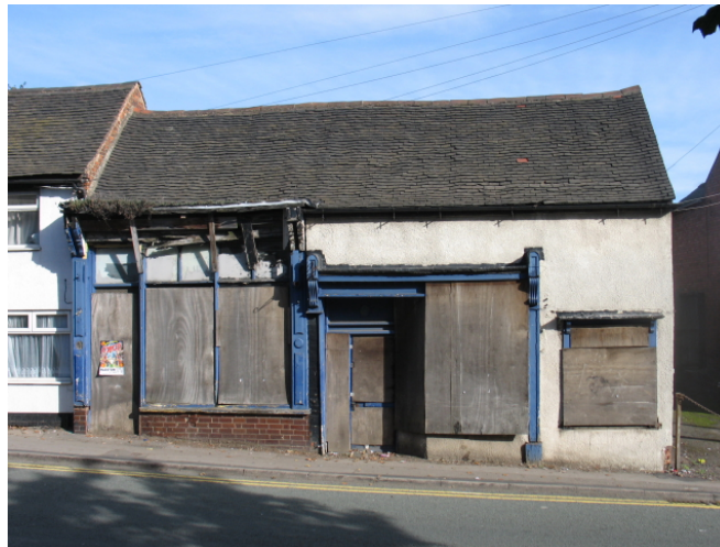
No. 36 Watling Street, in need of renovation
