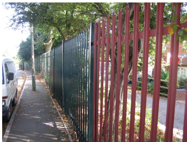
Inappropriate steel railings in front of Nos. 26-30 Glascote Lane
